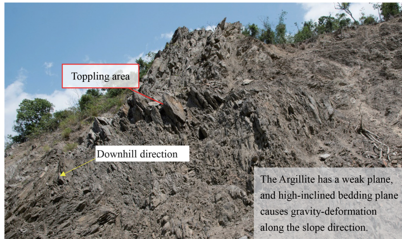
Fig. 3. An example of toppling area at the gully slope.
