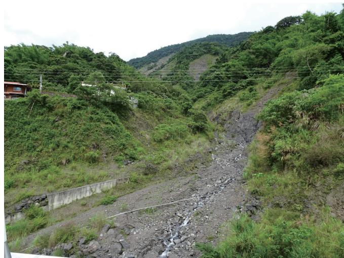
Fig. 5. The eroded material at the downstream of the erosion channel.
